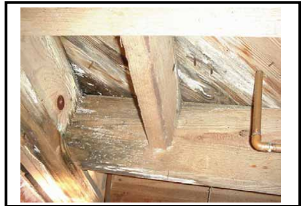
WATER LEAK UNDER MASTER SHOWER NEEDS REPAIR.
