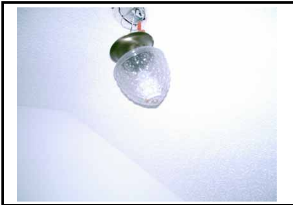
LIGHT FIXTURE IN BONUS ROOM IS NOT ATTACHED TO JUNCTION BOX
