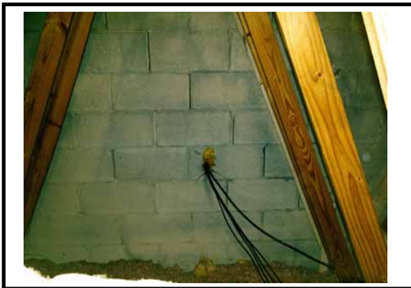
CABLE PASSAGE DRILLED THROUGH CONCRETE WALL IN BASEMENT NEEDS SEALED.
