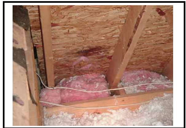
ROOF IS LEAKING IN LEFT REAR SIDE OF HOUSE AND NEEDS REPAIR.
