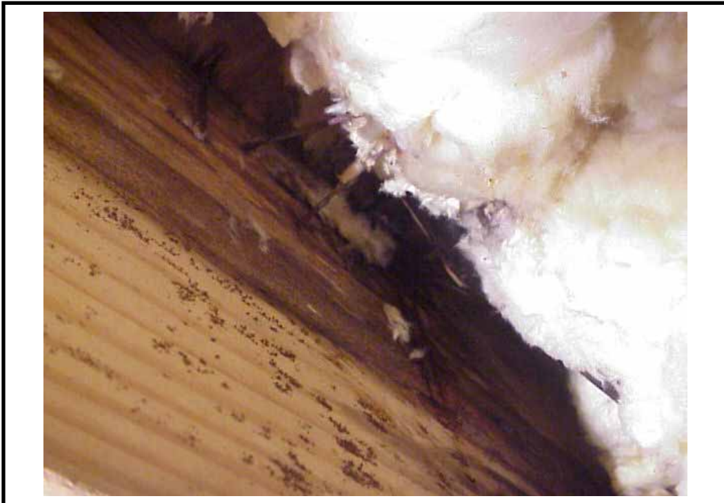
PICTURE OF LEAK UNDER THE MASTER BATH SHOWER
