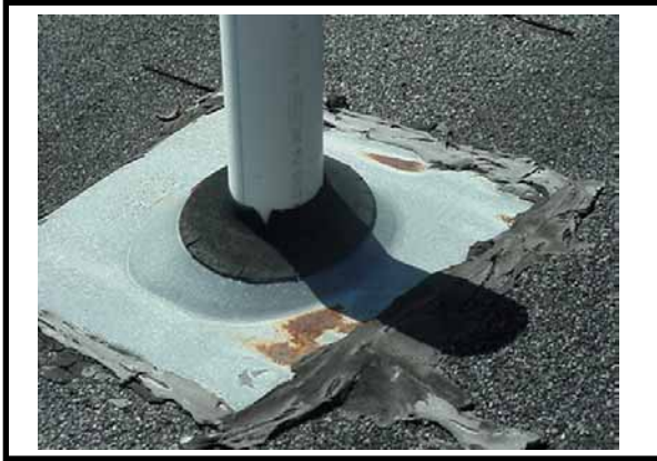
PLUMBING BOOT IS CRACKED AND NEEDS REPLACED.
