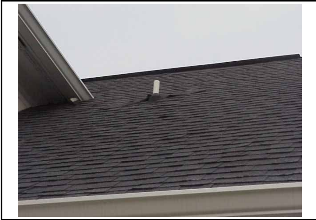
PICTURE OF LOOSE SHINGLE
