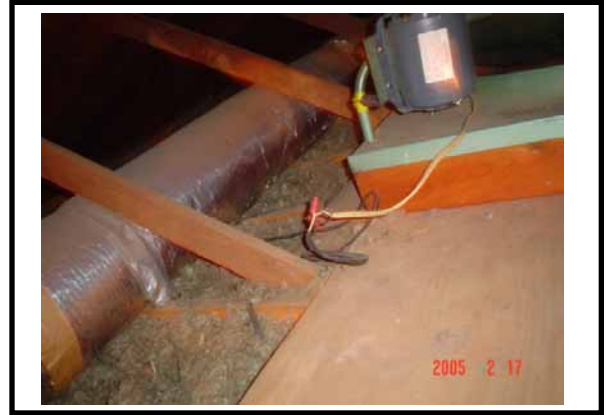
WIRE SPLICE TOWARD REAR OF THE HOUSE NEEDS TO BE PLACED IN A JUNCTION BOX.
